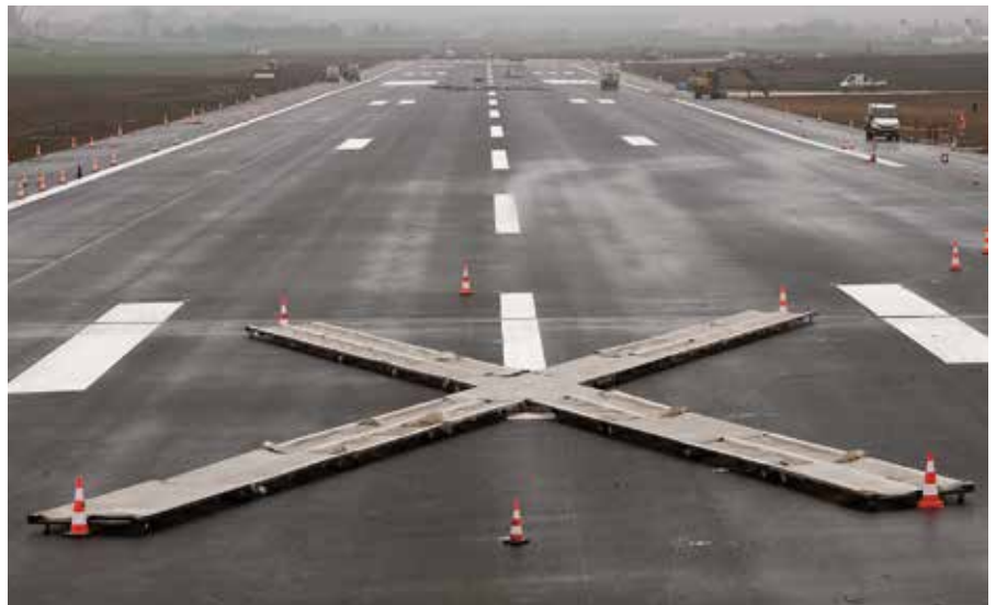
Paris-Orly: closure of the South runway for four months for rebuilding with a big impact on air traffic management.
