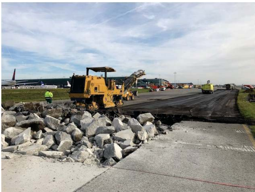
TAXIWAY ROMEO : rehabilitation of concrete surface and lights on 20 000 m 2 and creation of water drainage system
