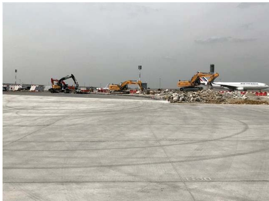
TAXIWAY TANGO: complete rehabilitation of surface course and lights on 24 500 m 2 (and 5000 m 2 taxiway shoulders)
