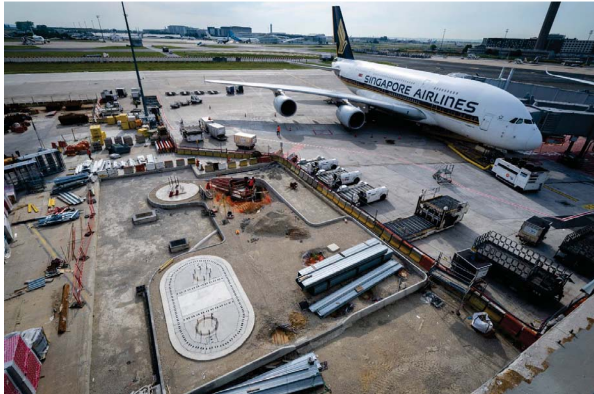
TERMINAL 1 JUNCTION – stand U11 Since June 2019
